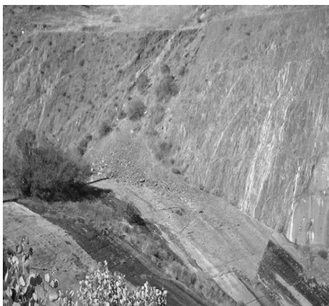
Fig. Slope failure at mountainous places
