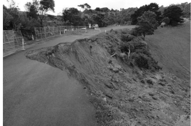
Fig. Slope failure at Highways
